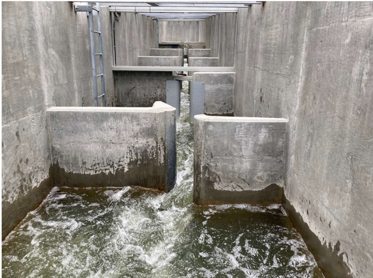
Figure 6-5. The BART Weir/ Rubber Dam 1 antenna in the fish ladder in Alameda Creek at river mile ALC9.67.
