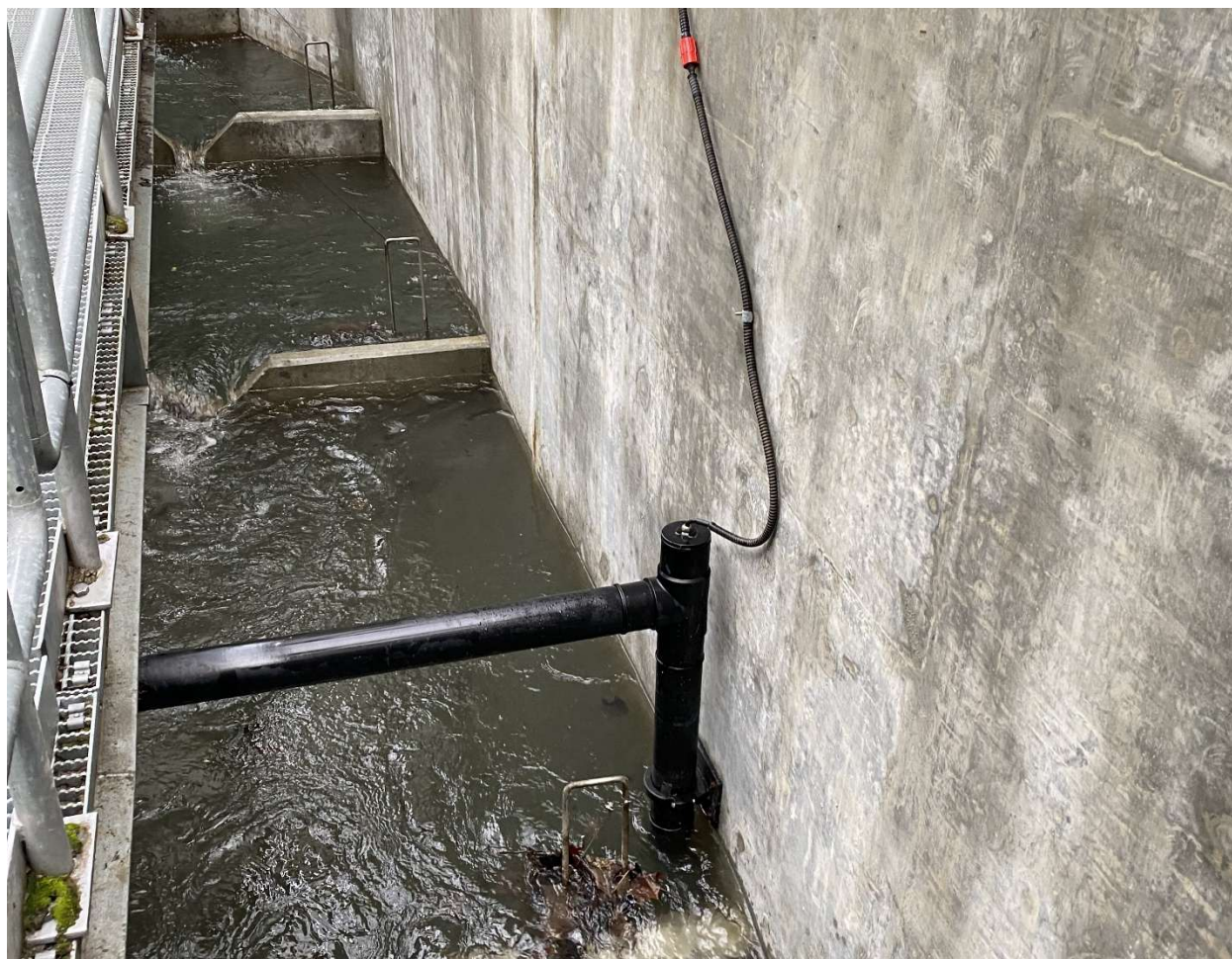
Figure 6-4. Biomark Passive Integrated Transponder tag antenna in the weir section of the Alameda Creek Diversion Dam fish ladder.
